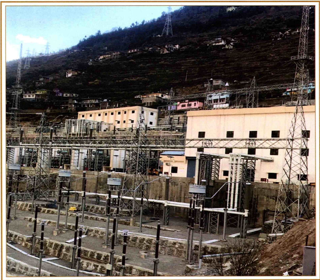
Lahal Sub-Station 400 kV, Chamba
